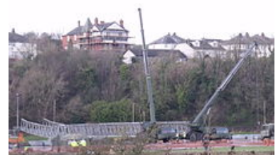
Sappers launching a Logistic Support Bridge at Workington in order to reduce effects of collapsed bridges
