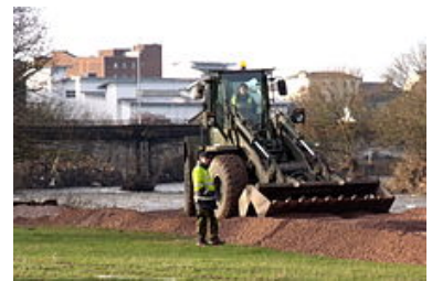
RE Plant Operators construct foundations for a new bridge in Workington after floods
